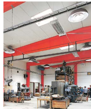
The temperature can be adapted perfectly in different areas of a room with IR. Spot heating increases the comfort and lowers the heating costs.
