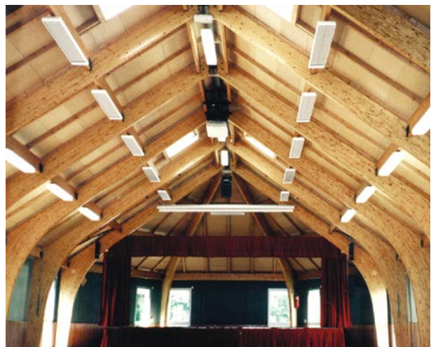
EZ200 gives instant heat and no preheating is necessary which makes it ideal for buildings that are used on an irregular basis.
